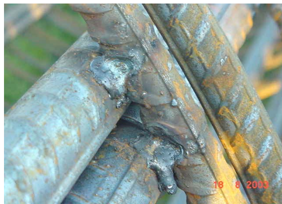
Figure 9. Example of Unacceptable Tack Weld Unacceptable weld width and undercut
