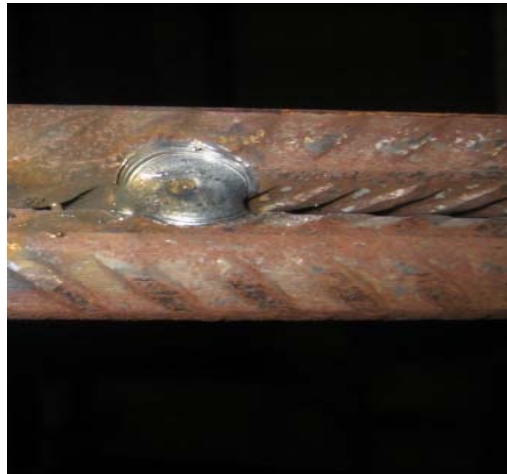
Figure 5. Example of Unacceptable Tack Weld Inadequate weld length
